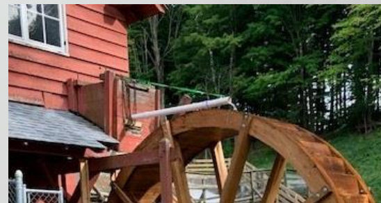
Our current, temporary flume is a PVC pipe supported by a ratchet strap.
